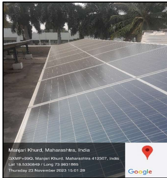
Photograph of Roof Top Solar PV Plant:
